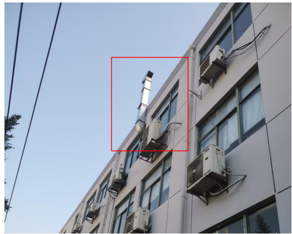
DA002 (TA003 处理后废气排放口)
